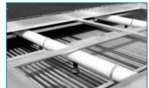
Drift Eliminators Removed for Coil Inspection
