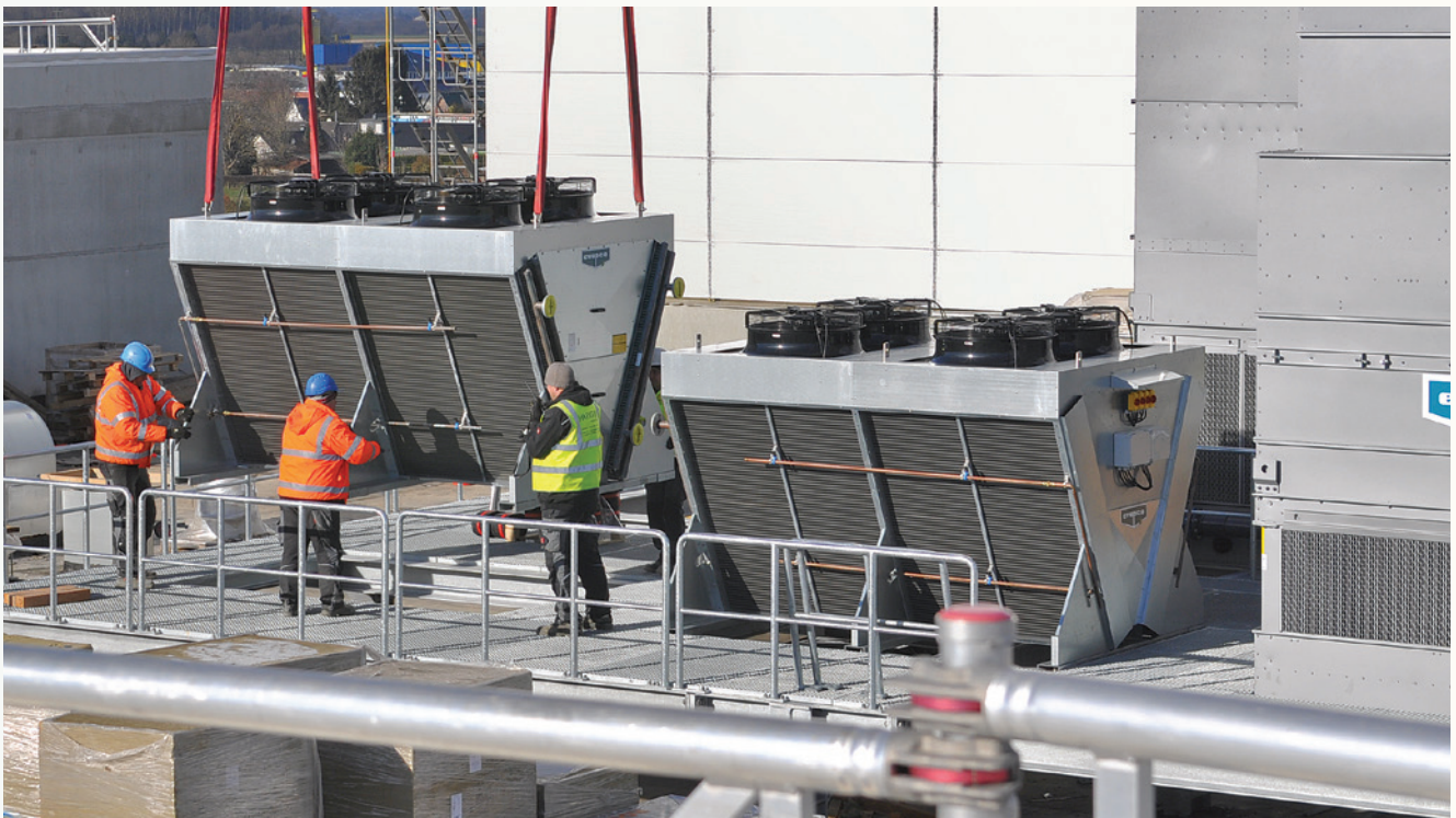
EVAPCO Air Solutions V Series, Germany
