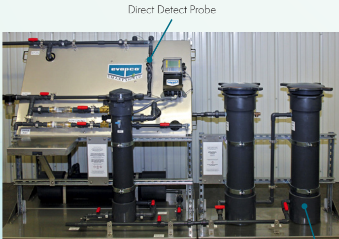
Monitored Release System
