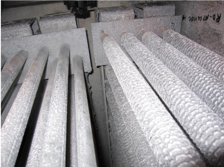
Commencement of Scale Formation on Both Coils
