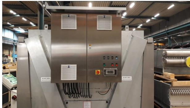
HMI, VFD and Bypass/ Off/Auto Switch for NEMA Motoren
